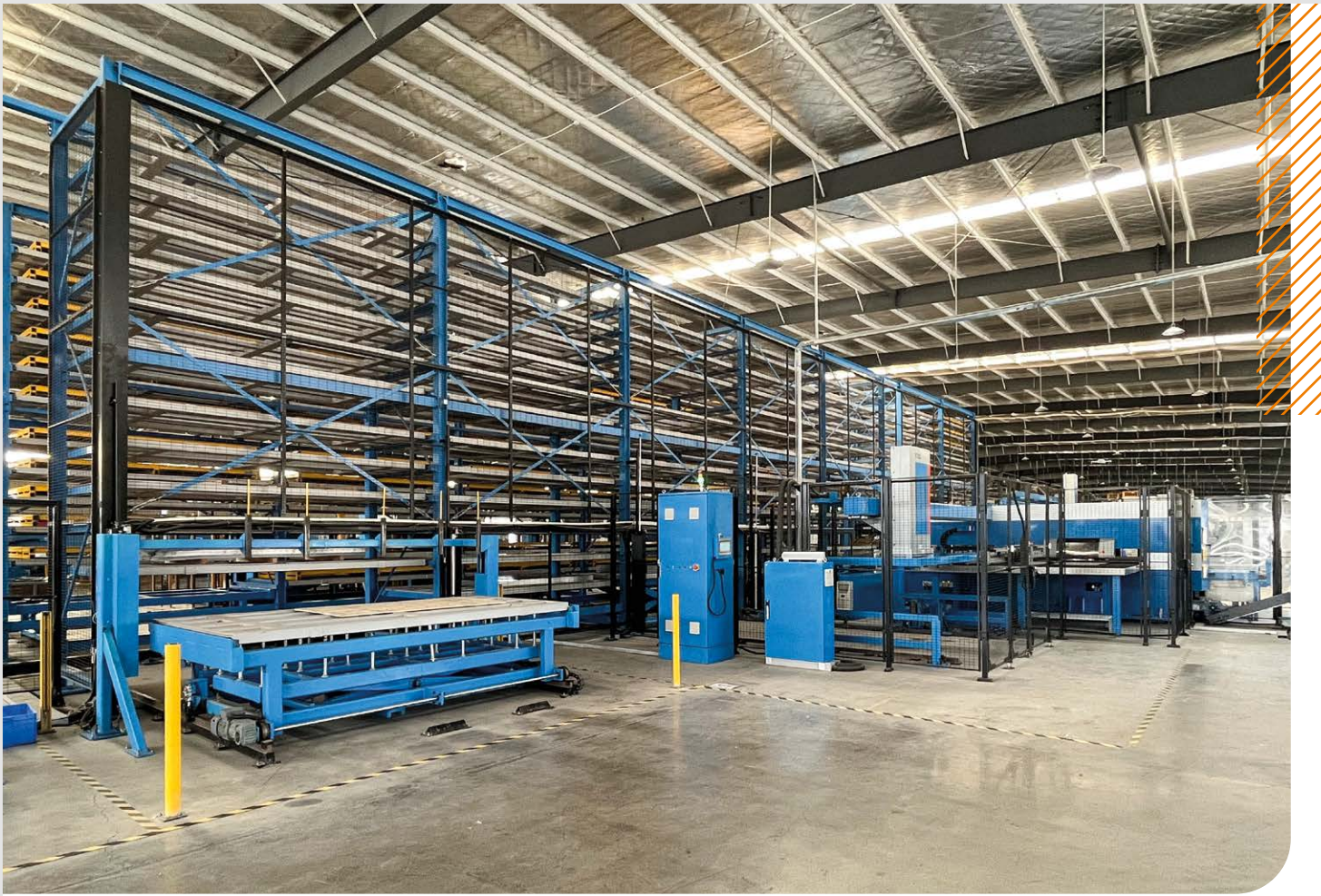
The Prima Power manufacturing line installed at Zhilai is connected to the Night Train FMS® automatic storage.
